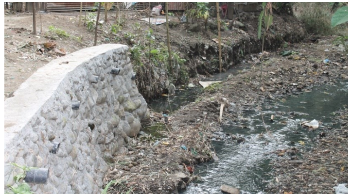
Figure 7. Unfinished rip-rap at Purok 2.
