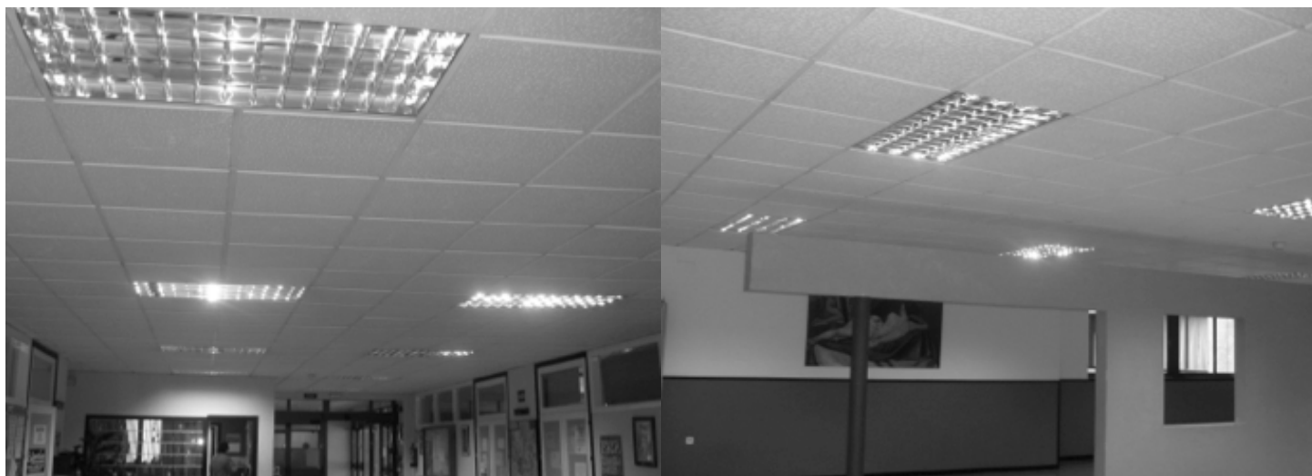
Figure 7. Recessed luminaries on the ground floor.
